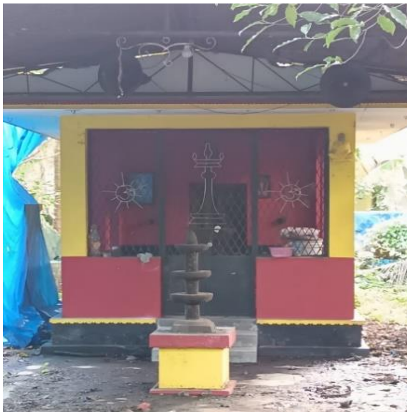
Figure 13 Front view of deteriorated sacred grove
